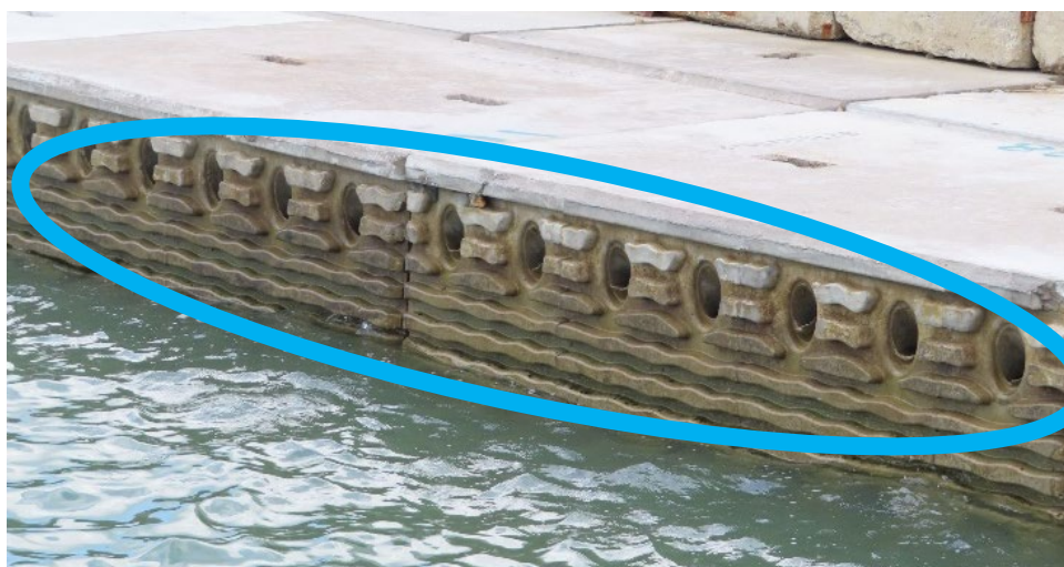
Example: Vertical Eco-shoreline at Tung Chung (eco-tiles)
